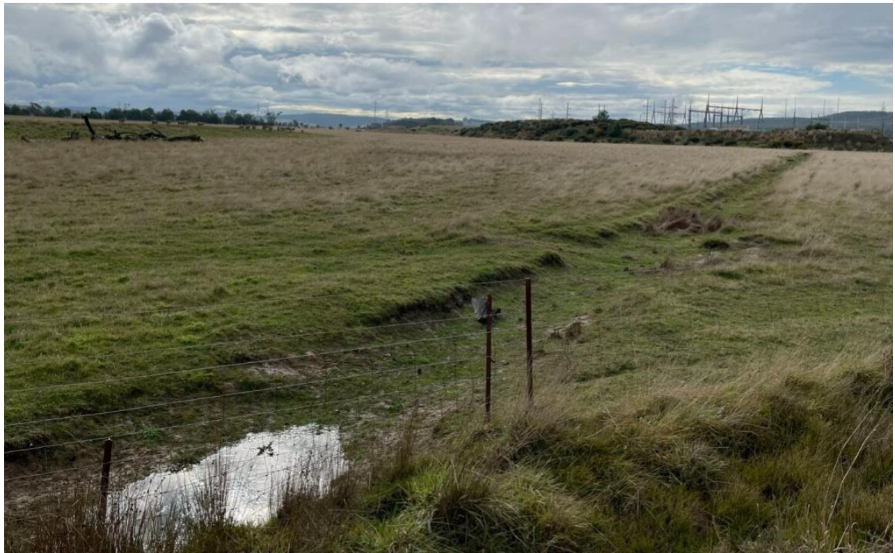
Figure 11: Open drain at its intersection with the road reserve looking north east towards the existing terminal station
