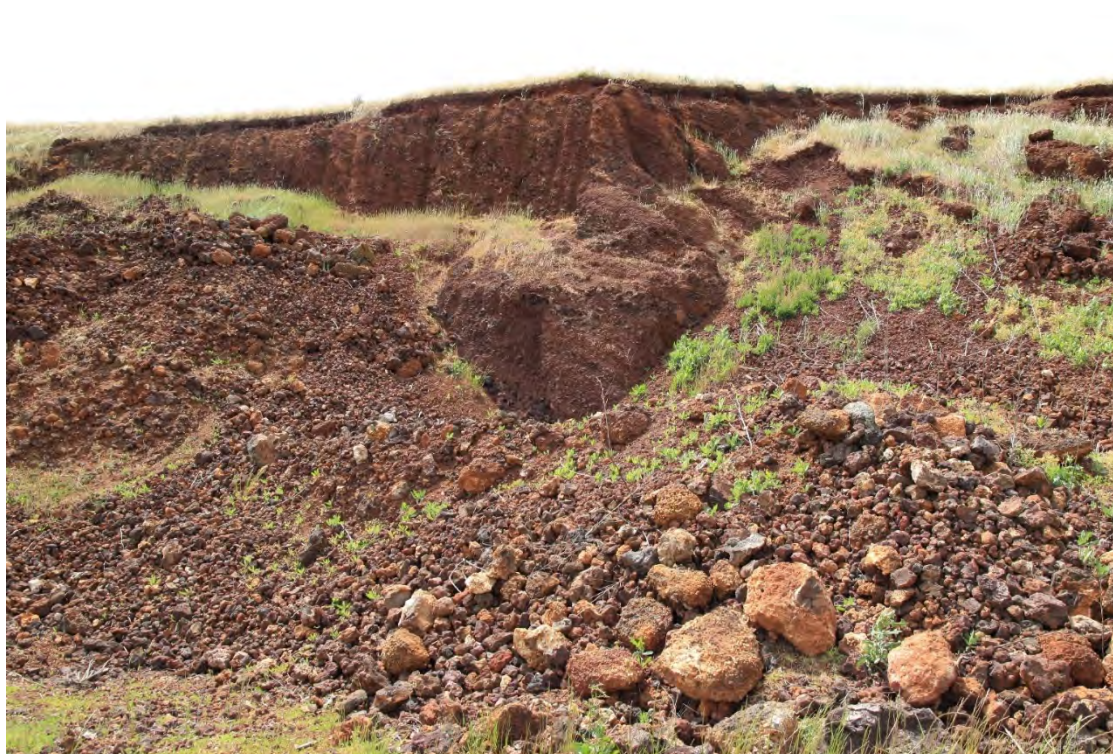
Photo 5 Mondilibi Hill quarry face; loose and consolidated scoria observable in the face
