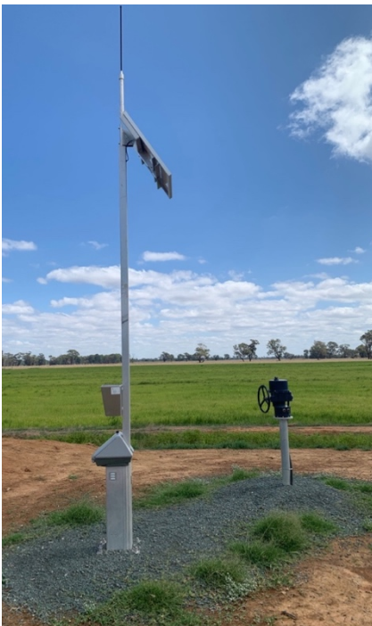
Figure 3-4: GMW service point
