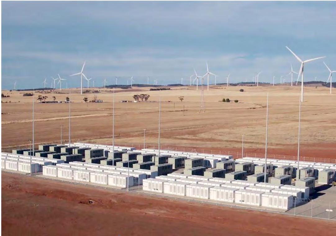
Plate 3 – Typical battery storage facility
