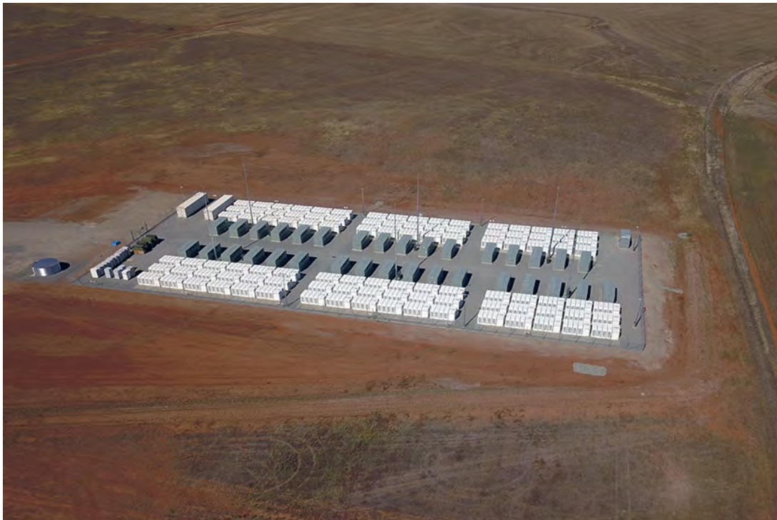
Plate 4 – Typical battery storage facility
