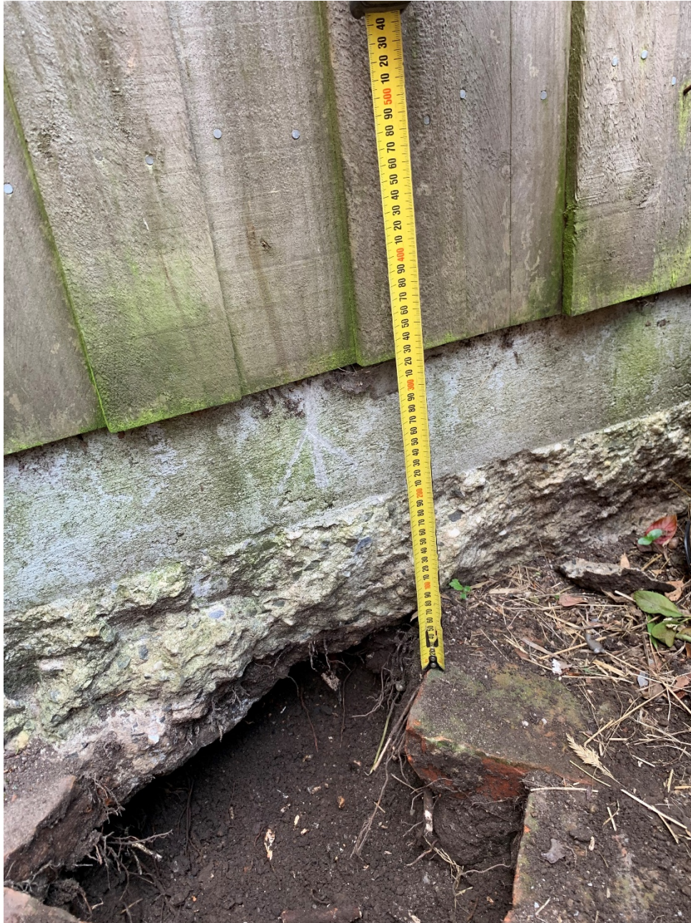
Figure 4. View of concrete footing, St. Patrick's Parish Primary School. (Ashley Wiseman, November, 2021).
