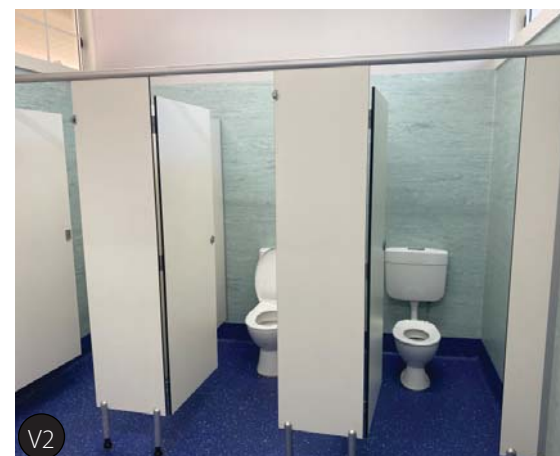
Dated partition system, fixtures & finishes in boys toilets.
