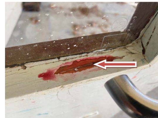
Door frame Classroom 1 – pink confirms presence of lead paint
