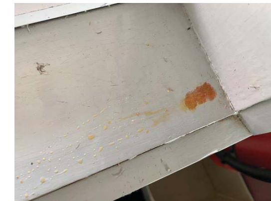
Internal window frame Classroom 4 – inconclusive part pink/yellow
