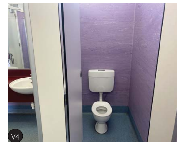
Inadequate layout of facilities.
